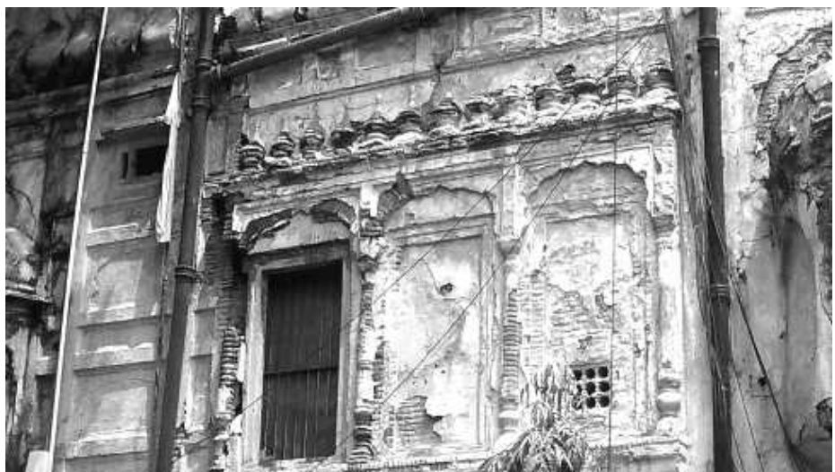
Figure 13: Damage to the ‘Service Club’ due to neglect, misuse and abuse.
