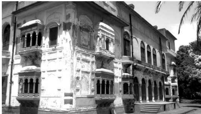
Figure 8: The Summer Palace during restoration, layers of plaster were peeled off to reveal original details.
