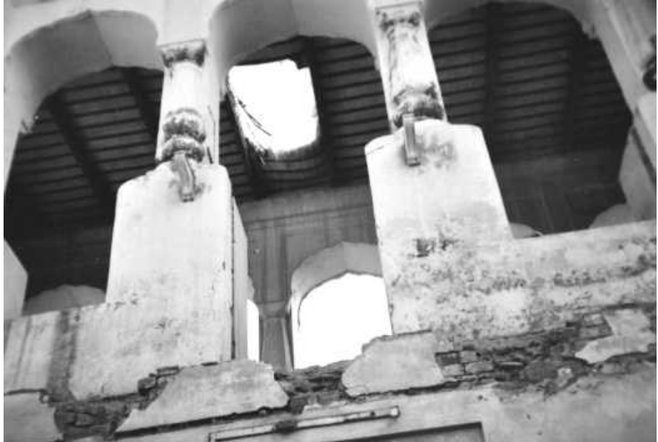
Figure 16: Damaged interiors of the Eastern Munshikhana
