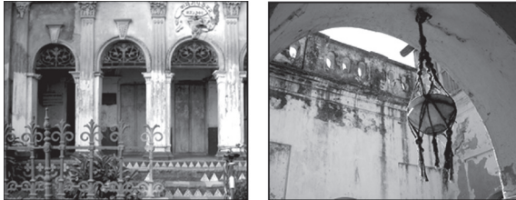
Figure 27: Exterior and interior walls of Kashinath Bhaban that is plastered with cement mortars is need to de-plaster. (Source: Photographs taken by the authors).
