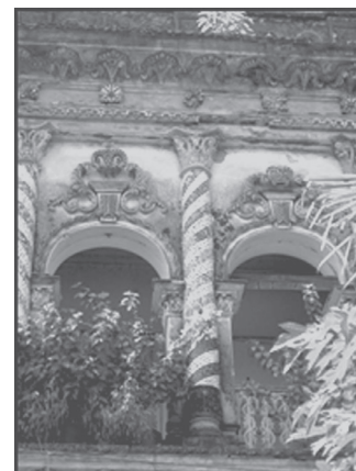
Figure 13: Plaster decoration and chinitikri work of the front facade. (Source: Khondker, S.M., July 2013).
