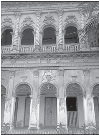
Figure 25: At present, front view of Kashinath Bhaban. (Source: Photograph of 2016 by authors).
