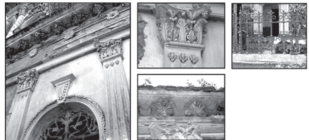
Figure 31: Some missing attributes, such as floral ornamentation, cast iron railing etc. (Source: Photographs taken by the authors).
