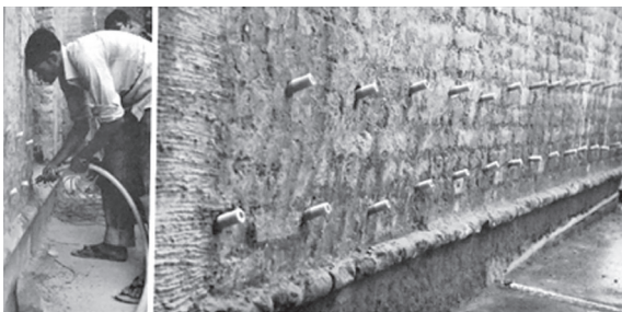
Figure 28: An example of insertion of damp proof course (DPC) into the existing wall. (Source: Ahmed, 2015).
