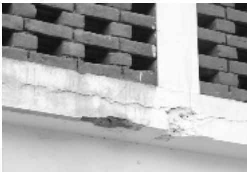
Figure 13 (Bottom Left): Rusted and weathered reinforcement can be seen wherever concrete cover has come off.
