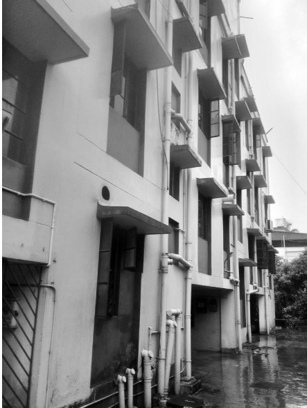
Figure 1: Entry to Phase I flats remains submerged in water all year round, making access to flats difficult and hazardous.
