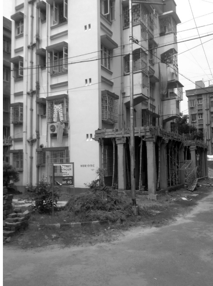
Figure 2: Extension work and covering of balconies in Phase II flats makes rooms dark and stuffy, and unsuitable for healthy living.
