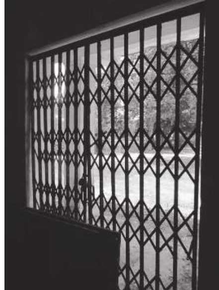
Figure 32. Collapsible door which was earlier act as a main entry to the stadium. (Source: Clicked by Author).
