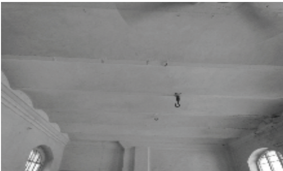
Figure 27. Vaulted ribs roof transferring the load to the huge walls. It's made by iron girders and bricks as a basic construction material (Source: Clicked by Author)..
