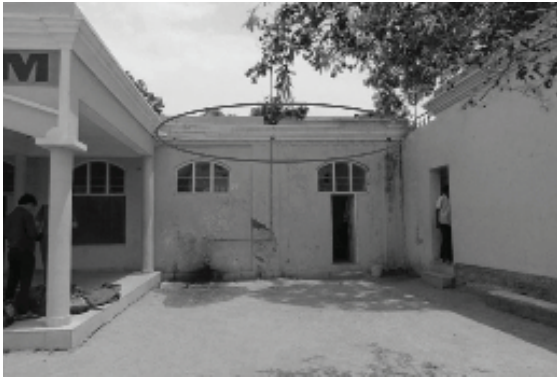
Figure 29. Cornice band is running at the top of the building (Source: Clicked by Author).
