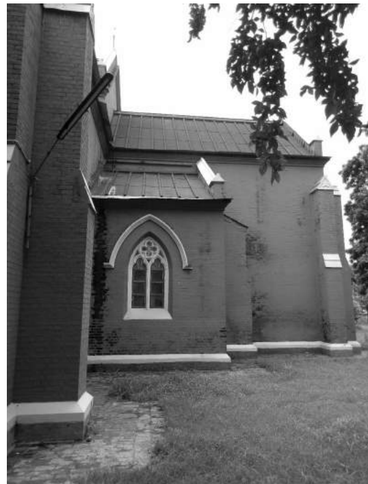
Figure 12. The walls with varying widths and GI sheets used to cover the roof trusses (Source: Author)
