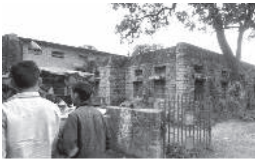
Figure 8: Dilapidated condition of Land Revenue office in Hamirpur town, H.P.
